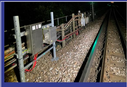
Immunisation transformers and capacitors installed and commissioned into service ready for Phase 2
